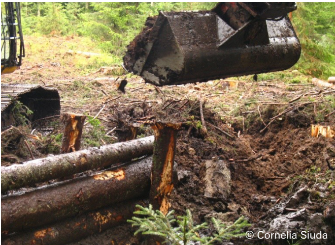
Construction with tansverse and vertical logs before coverage with peat and vegetation sods
