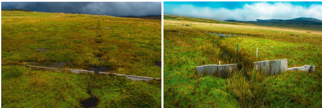
Pugllohuma Peatland: drain 5 years after blockage by wooden dikes. Napo Province, Ecuador © FONAG
