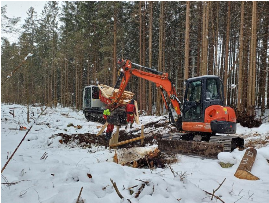
Picture: Installation of a sheet pile in Spirkenmoor close to Griesbach; © Sharon Rakowski und Kerstin Bär
