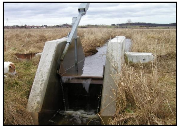
Picture: Adjustable dam in the southern Federseeried, which has promoted the acceptance of waterlogging and allows water levels to be adjusted.
