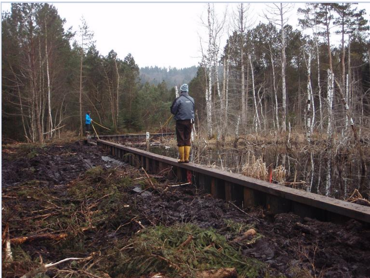
Picture: Peatland ecologist Cornelia Siuda and construction supervisor Axel Thiele on the installed steel sheet pile wall in the Eglinger Filz (© E. Pleyl)
